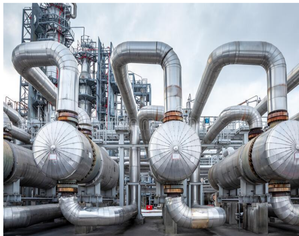
Figure 1: Three Shell and Tube Heat Exchangers
