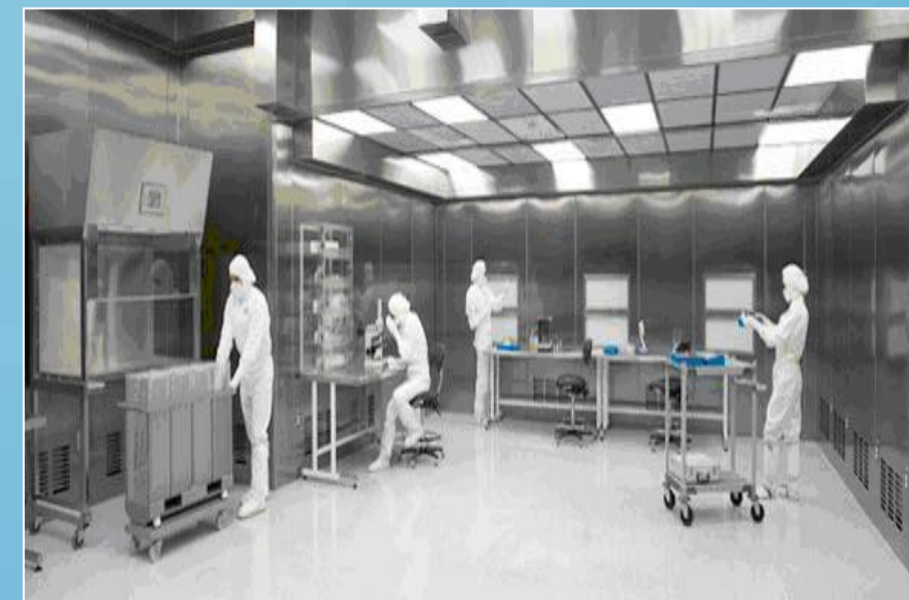
Figure 4 : Typical Cleanroom in a pharmaceutical Industrial Factory
