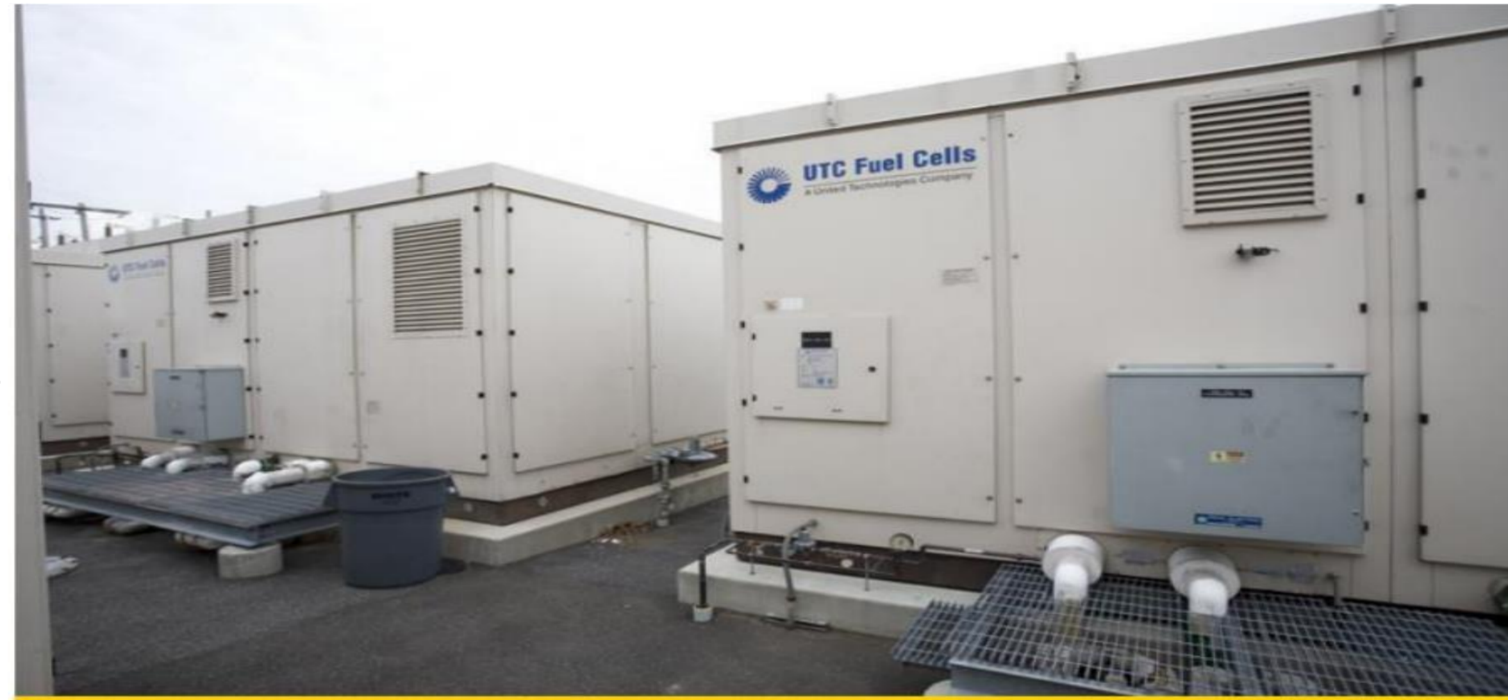
Figure 2: Phosphoric Acid Fuel Cell CHP System Installed at Verizon Central Office
