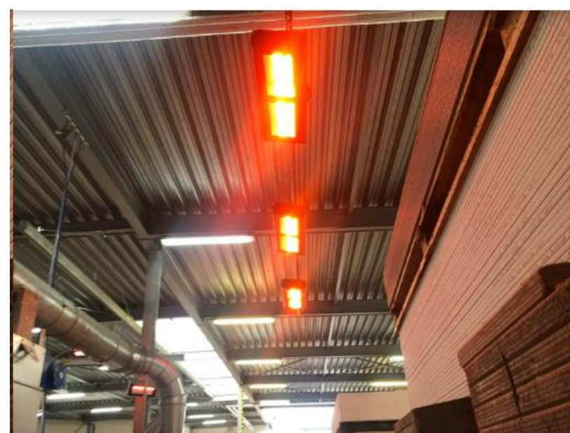
Photo of: Chain Hung Electrical Near-Infrared Heaters
